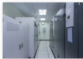
Uninterruptible Power Supply
