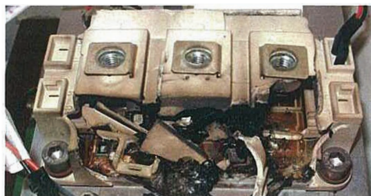
Figure 38: IGBT Case Rupture During a Short-circuit Fault Condition
